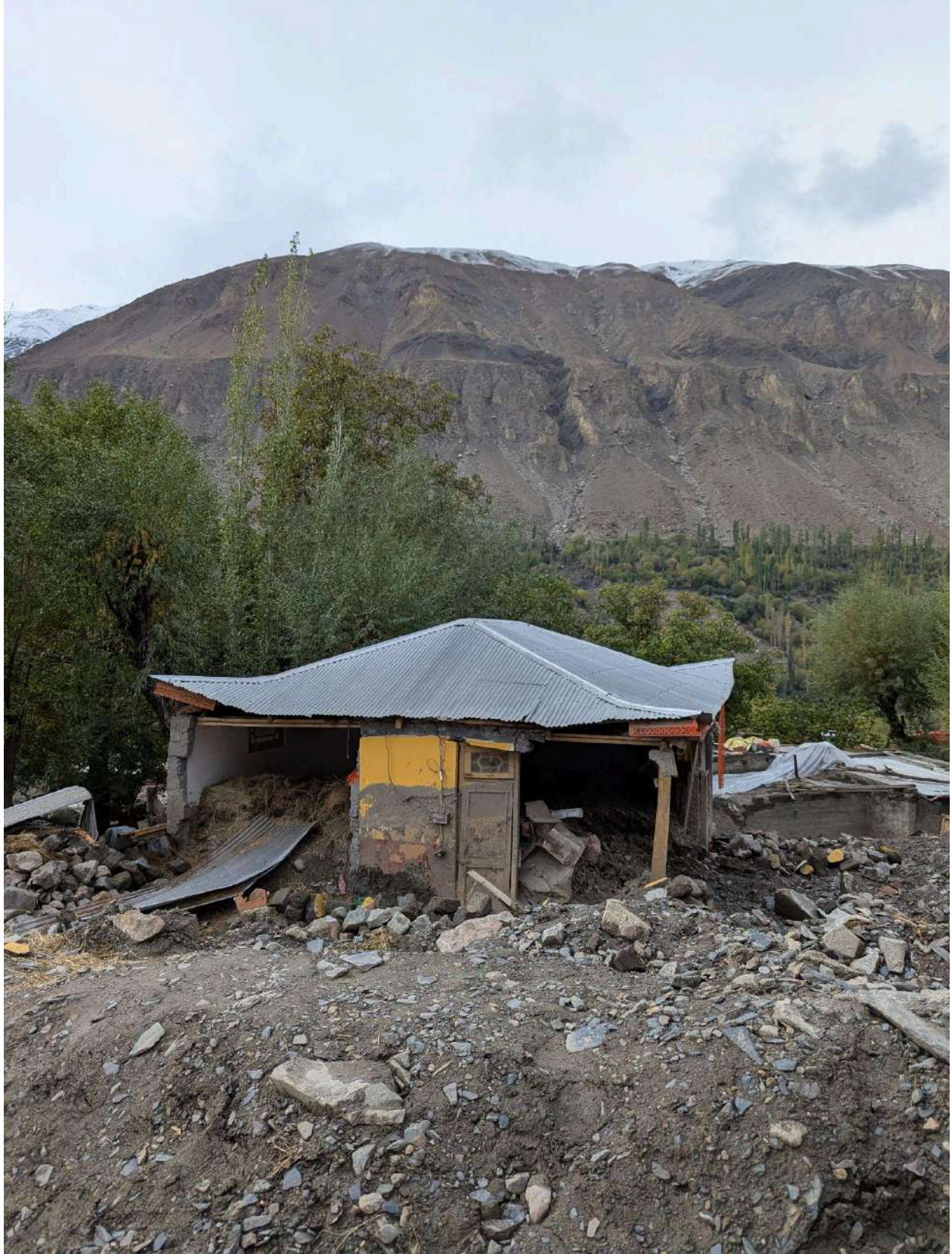
The aftermath of floods at Thui, Yasin Valley, GB
